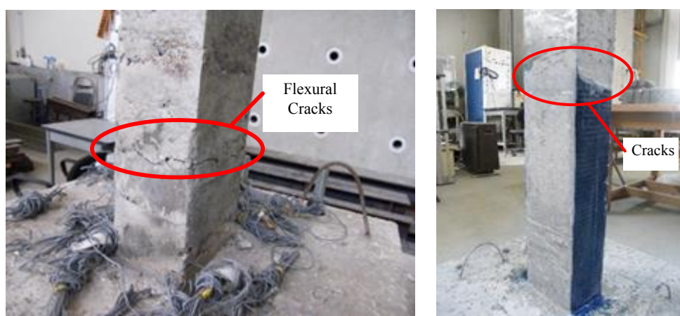
(a) Cracks in original specimen
