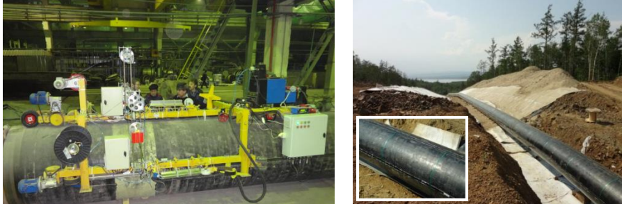
Figure 3: a) Automated machine for simultaneous integration of 3 sensors on a pipeline and b) example of field installation of 3D deformation monitoring.
