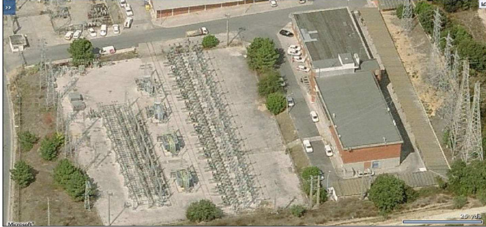
Fig. 3. Substation perimeter surveillance.
