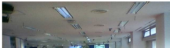
Fig. 4. Ceiling of the South Laboratory with installed sensors.
