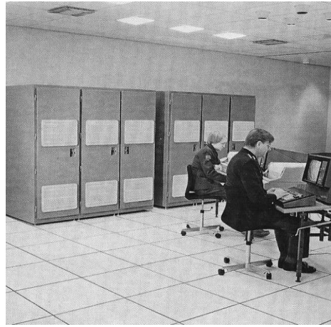
Fig. 7. Typical CAMPS Installation
