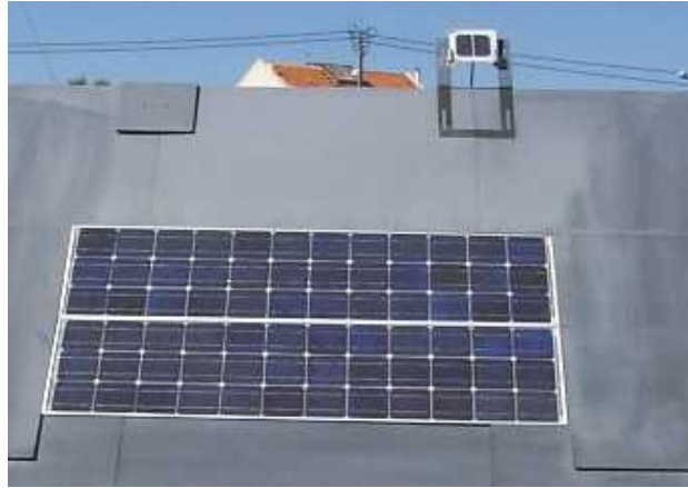
Fig. 4. PV system formed by two monocrystalline solar modules series-connected.
