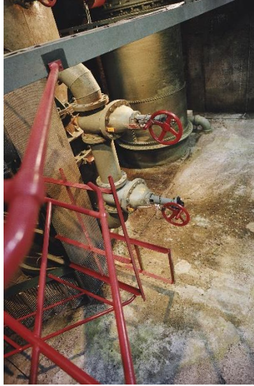
Fig. 4. Head valve of the Lau Balagnas hydroelectric power plant. (©EDF – Gilles de Fayet)
